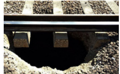
Sinkhole under railway tracks
